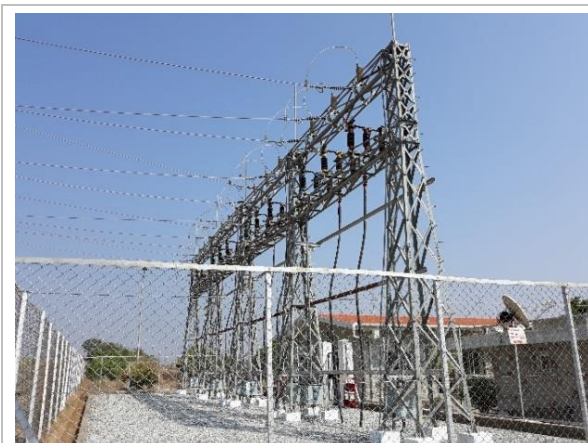
Detailed view of the gantry structure of the substation at which four circuits arrive from the wind farm (two double circuit lines).
