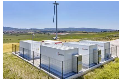
#1 Hybrid wind power storage plant in Spain using batteries
